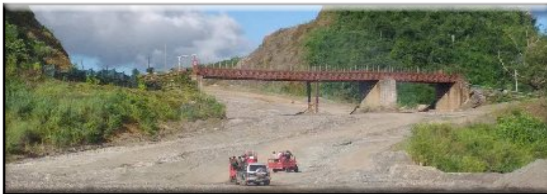
This bridge used to span the Gwihka Stream, which has now dried up due to mining
